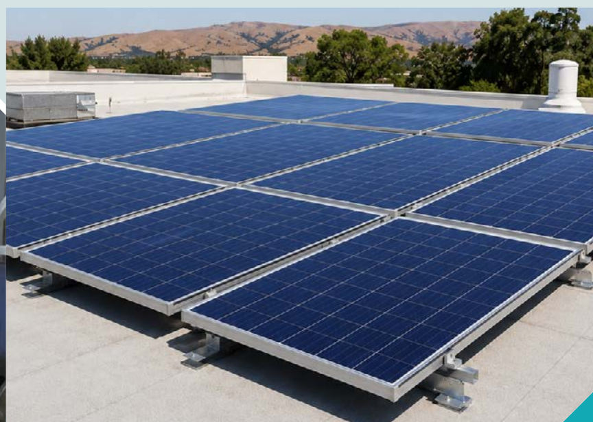
Residential solar mounting structures
